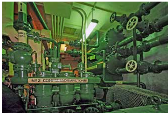
The air-conditioning plant room.
